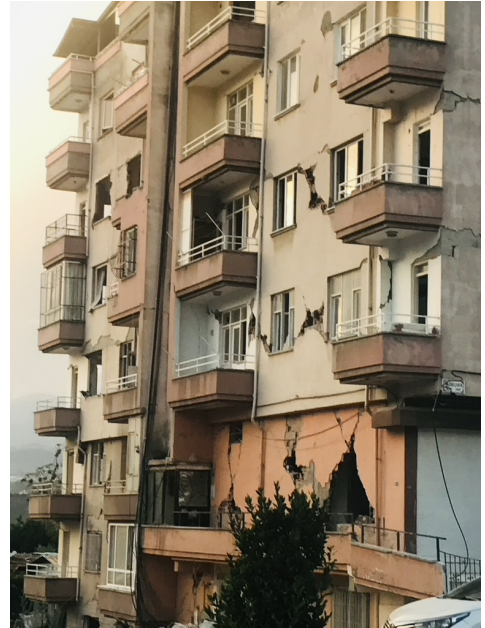
Homes destroyed by earthquake.
